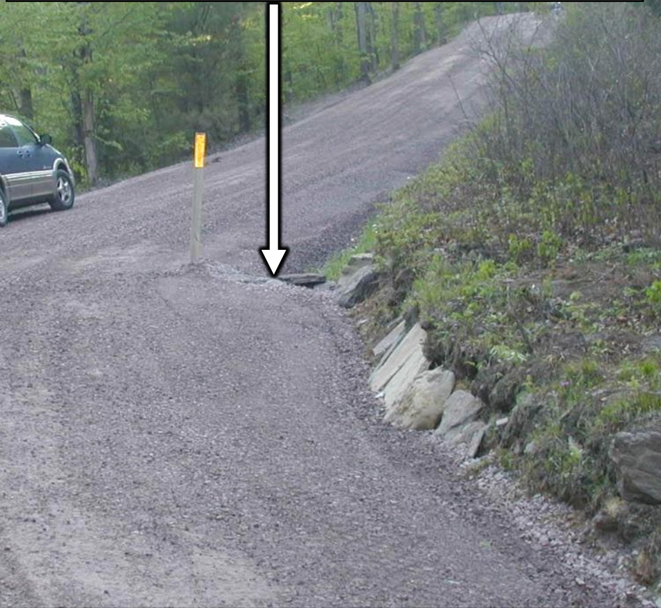
Before: Inlet too close to road
