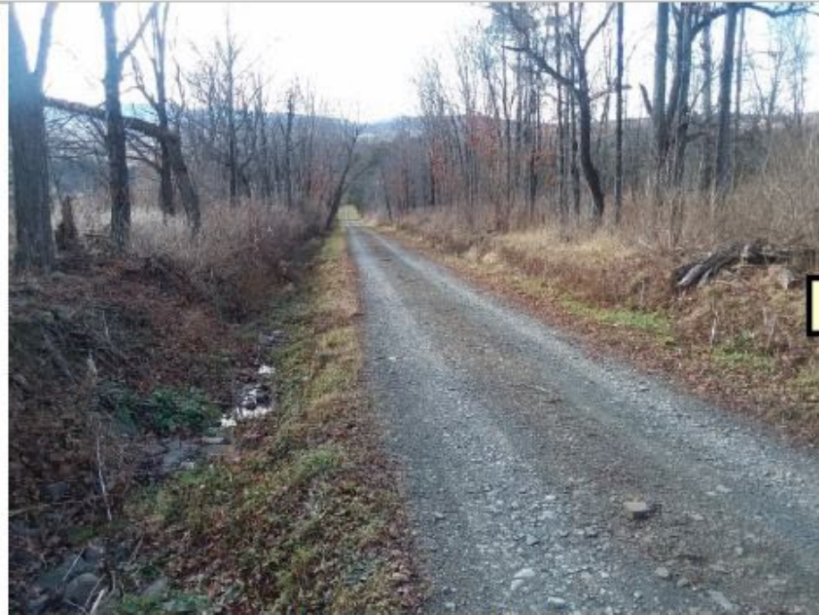
BEFORE: Top of hill is entrenched and channeling water
