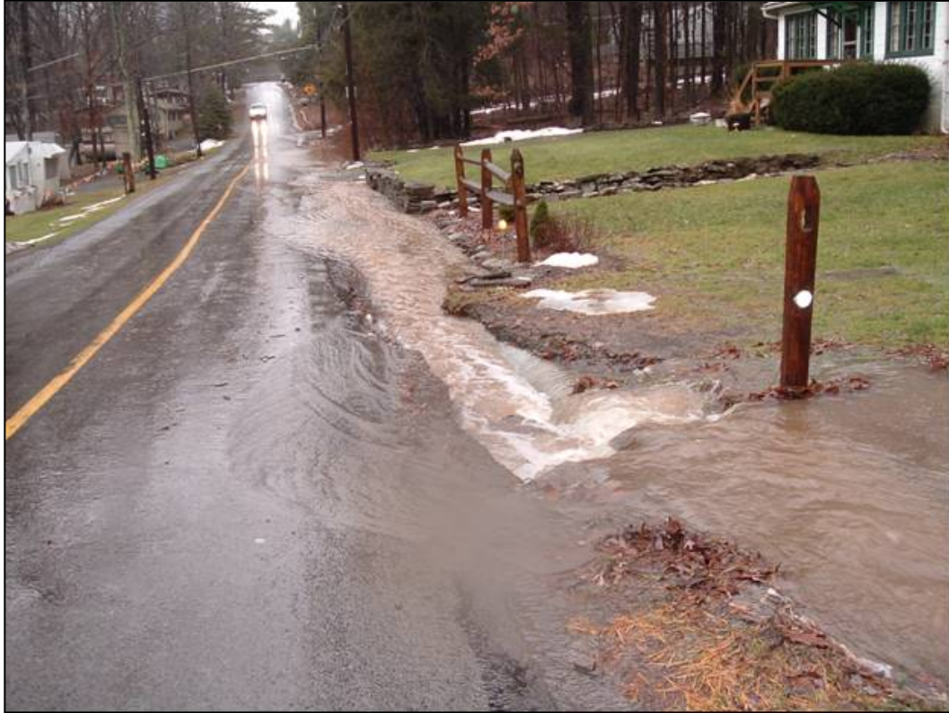
Roadside and Flooding during rain event before BMPs installed
