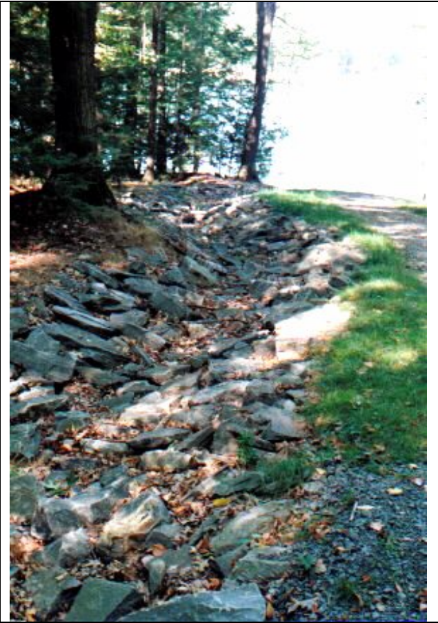
Rock-lined channel designed to reduce stormwater erosion along roadside in Paupack Township
