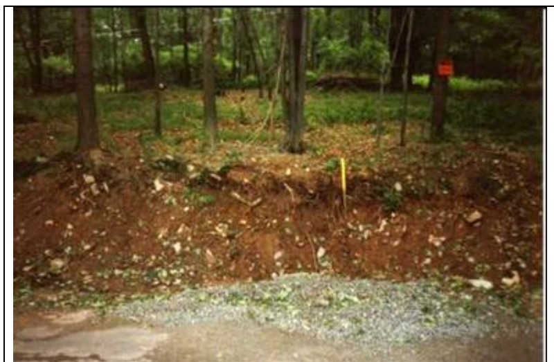
Roadside bank erosion problem area
