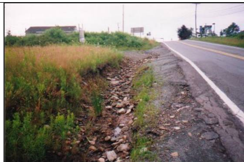
Roadside in need of repair and stormwater management
